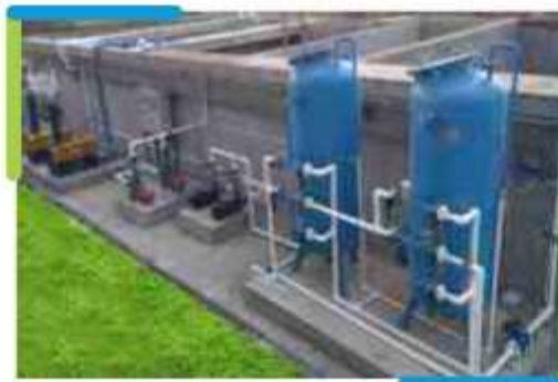
Conventional Sewage Treatment Plant 10 KLD – 2 MLD
